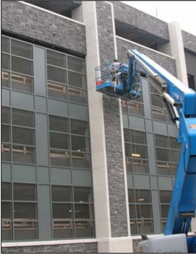
LEFT: Installers put finishing touches on stone panels at Fordham University's parking facility.
