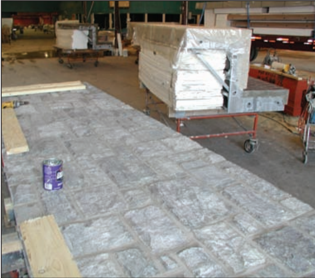
LEFT AND OPPOSITE RIGHT: Construction detail of thin veneer panels being assembled at EEWS facility in Bethlehem, Pa.
