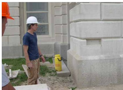
Eric Kudrna points out a Dutchman patch at the Kansas State Capitol restoration project.
